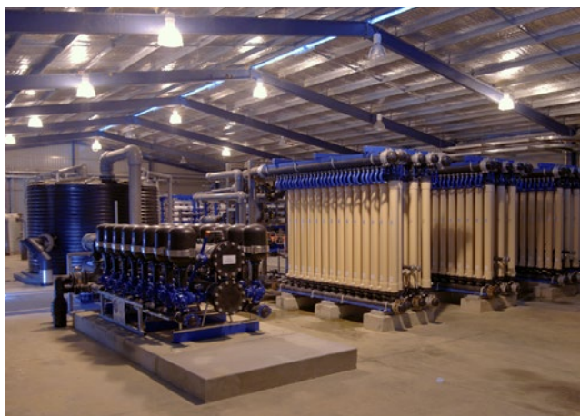
Figure 1. Water treatment plant (photo source: Australia Pacific LNG).
